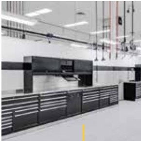
Service Bays & Toolboxes
